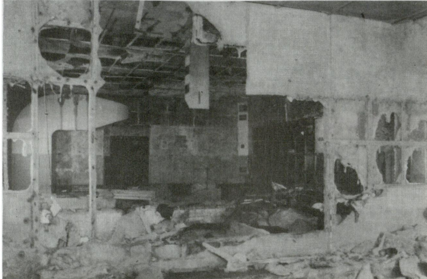
Photograph 8 Disused underground radar station at Wartling (Kent) lit entirely from hidden flash positions
